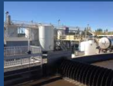
Secondary wastewater treatment (WW)
